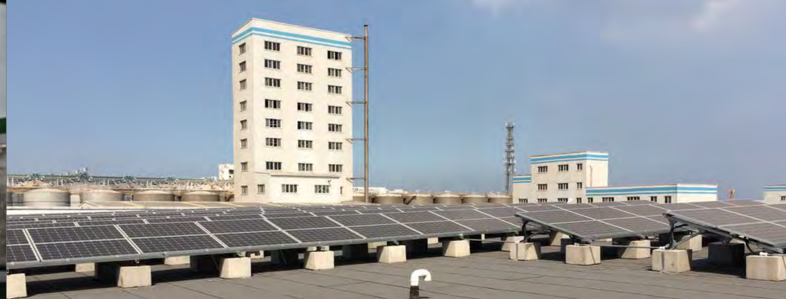
New solar panels at our oilseeds processing plant in Tianjin, China
